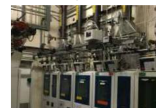
Linear Technology Silicon Valley FAG Gas Supply System Control - USA
